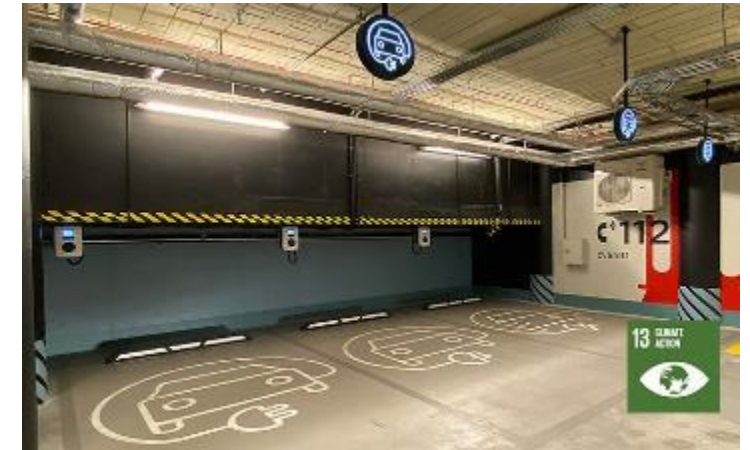
Electric vehicle charging
